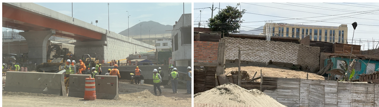
Figure 7: Construction of new roads for the port at Chancay (left); view of the COSCO administrative offices as residents are displaced (IBI Consultants, November 2024)
